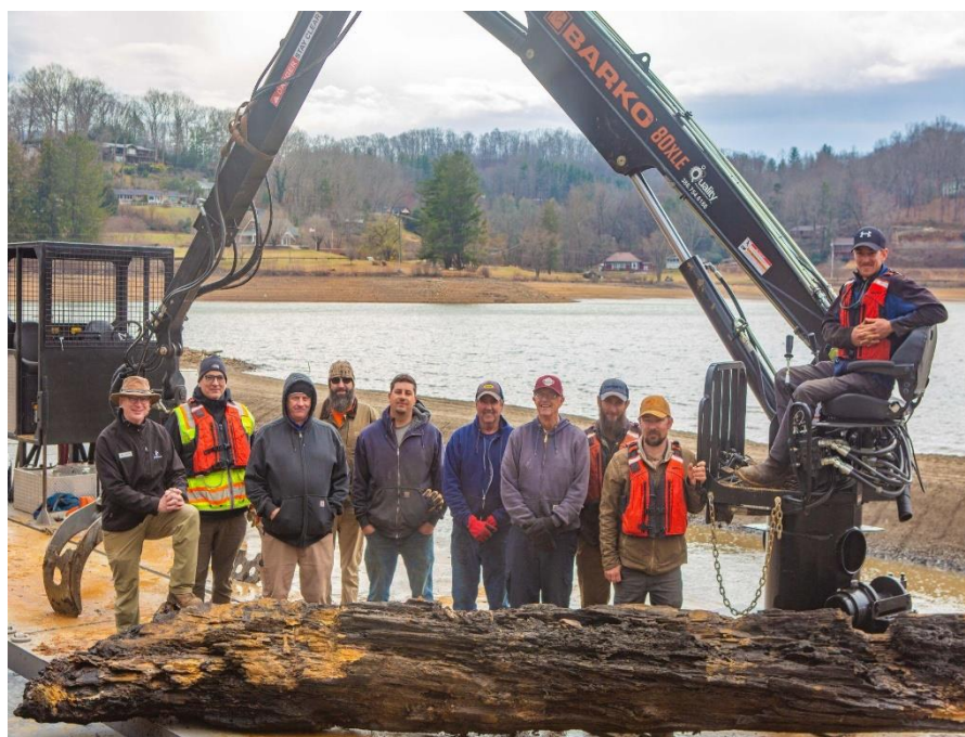
From left, Ken Howle, executive director of Lake Junaluska Assembly; John Garner, principal Garner Engineering; Carroll Woody Jr., director of Lake Junaluska's Assembly Public Works; Brian Aldridge, Trevor Cool, Danny Trull, Mackie McKay, RCF Construction; Adam King, owner, Crestline Global; Patrick Fish and Philip King, owner, Crestline Global.
